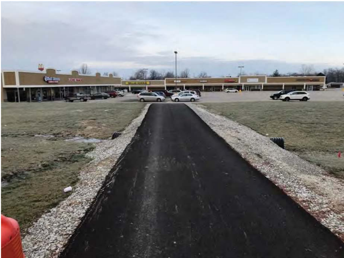
38. Looking W at intersection of proposed trail and existing path E of Linton Shopping Center
