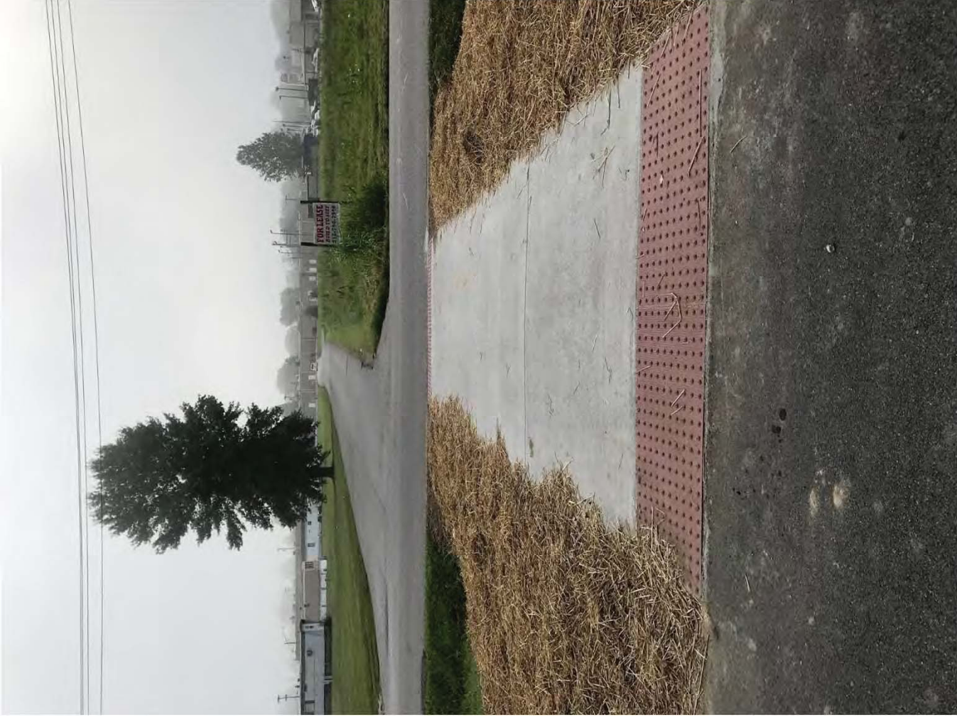
Looking E at the newly constructed sidewalk at the intersection of CR 1100 W and the unnamed access drive E of Humphreys Park
