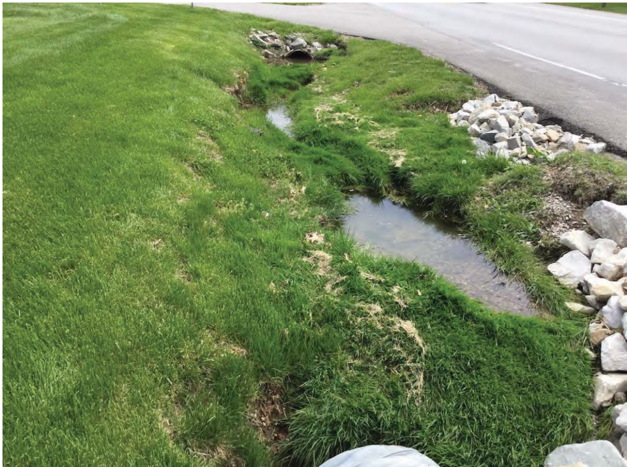
32. Looking east along UNT 5 at failed culverts
