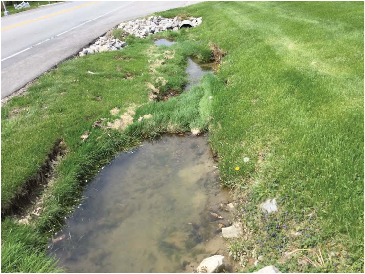
33. Looking west along UNT 5 at failed culverts
